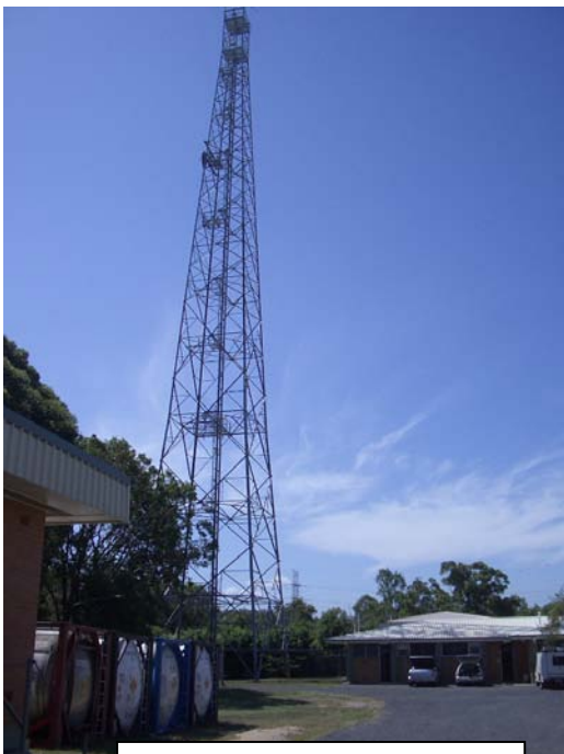
Communications: lattice frame
